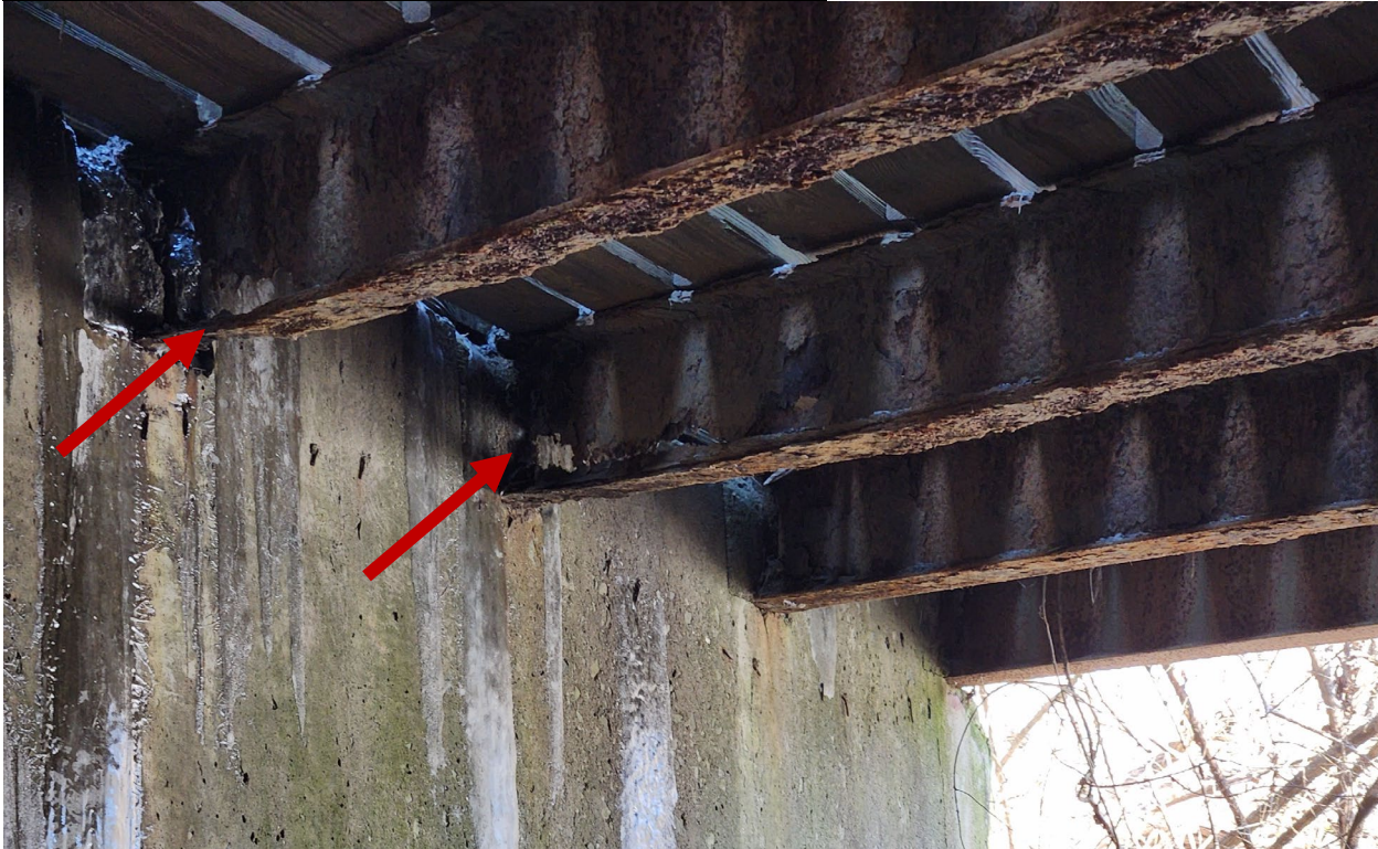
Holes in Two Steel Beams at the Northwest Abutment
