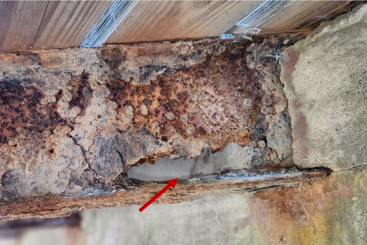
Extreme Corrosion and Hole in Steel Beams at the Southeast Abutment
