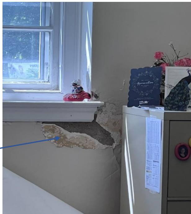
Figure 4. Interior water damage.
