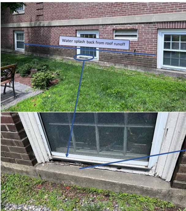
Figure 3. Water damage from roof runoff.
