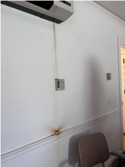
Figure 1. Planning and zoning condensate damage from air conditioning systems.
