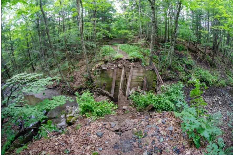
Collapsed bridge severed the Norwich trails network. (Photo D. Hardy)
