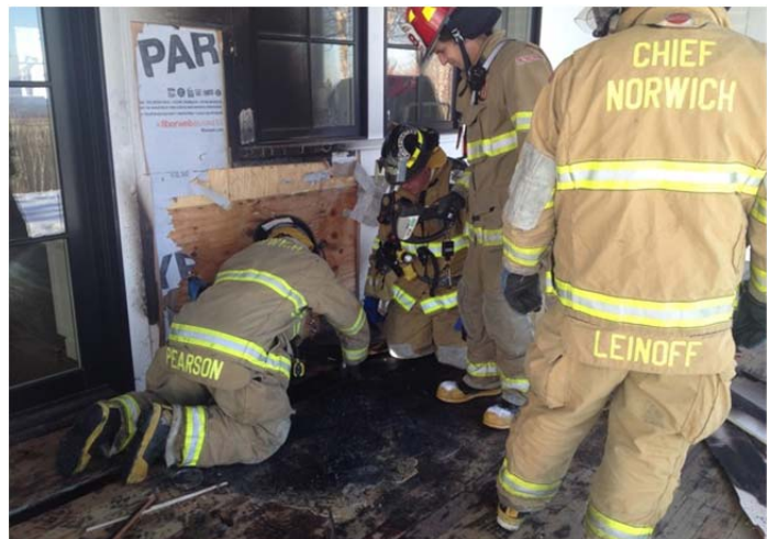
Members removing burned materials to check for fire extension at Birch Hill Lane.
