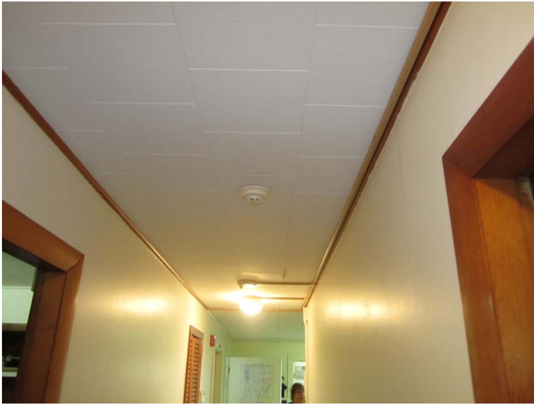
Photograph No. 7: Flammable ceiling tile typical throughout the building.
