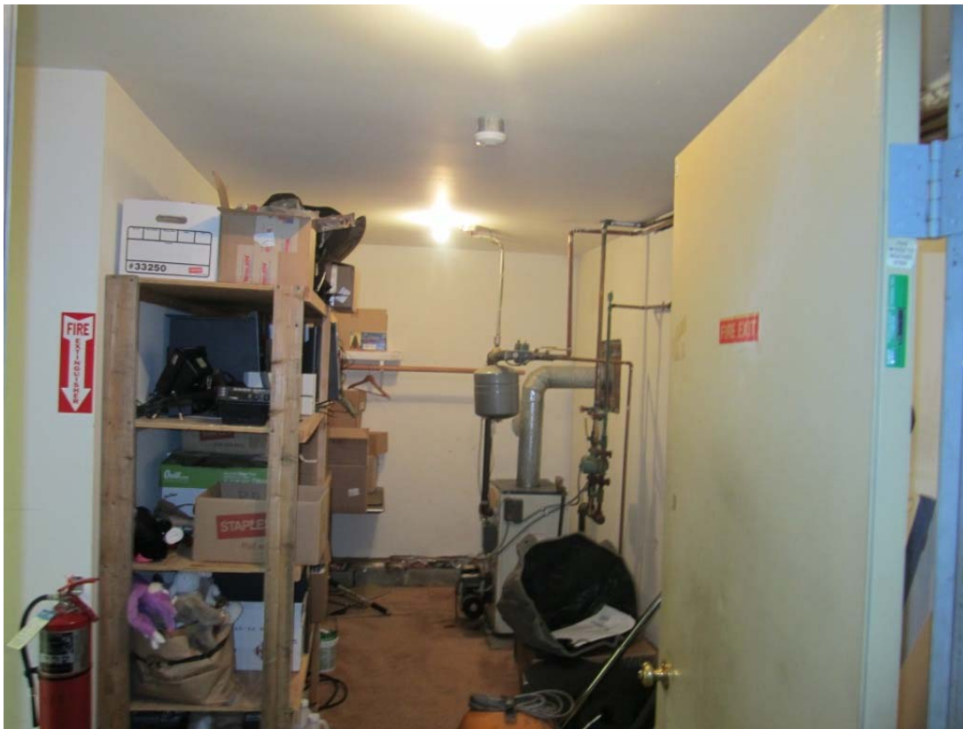
Photograph No. 11: Furnace room with open storage.
