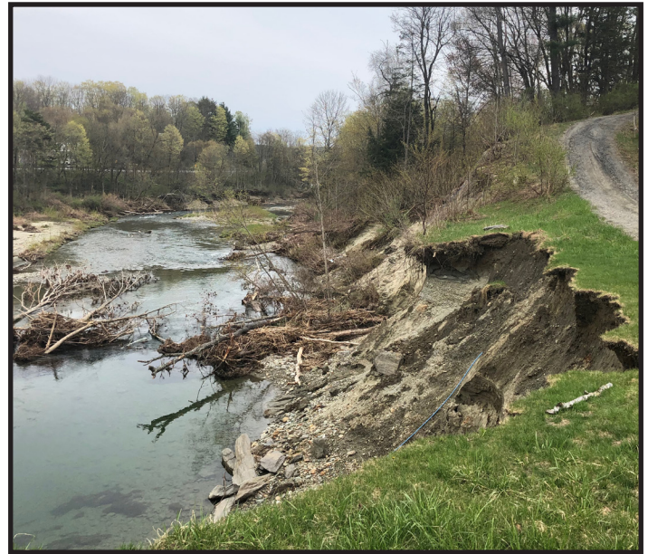
Streams and rivers can have tremendous erosive force when large volumes of water are moving at high velocity. Streambank erosion can put roads and homes at significant risk.
