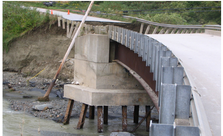
Damage to a bridge following Tropical Storm Irene
