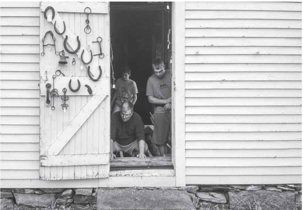
Norwich Scouts led by Joe Porter build a new floor for the Historical Society's tool shed as a community service project.
