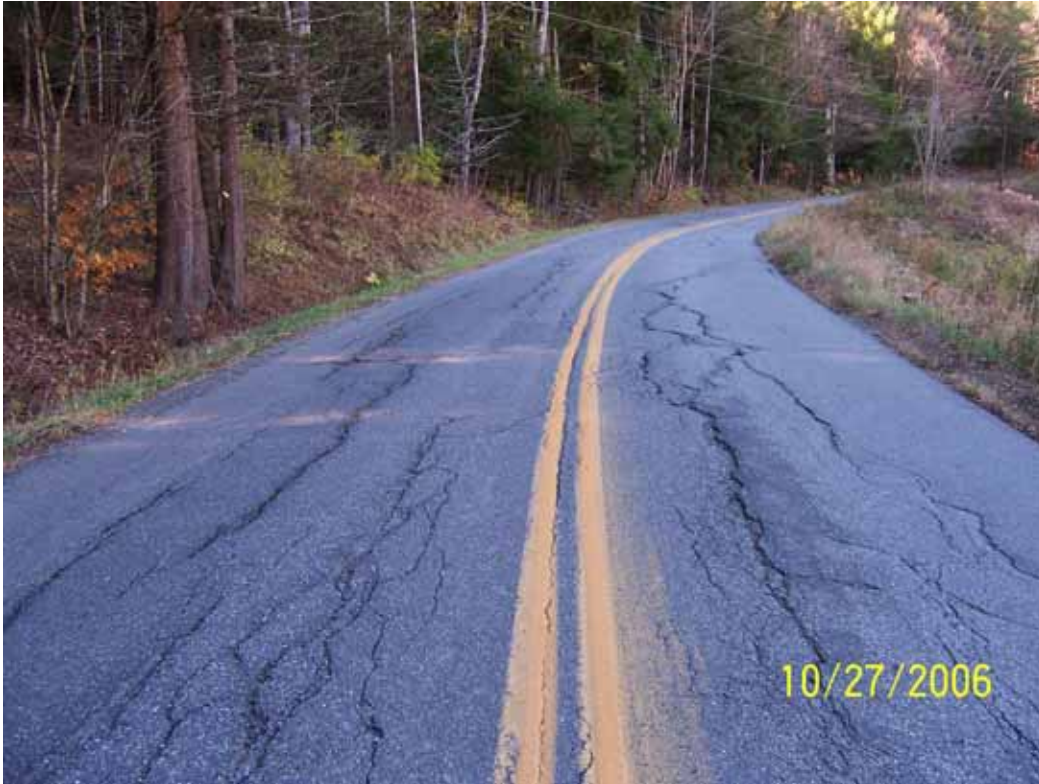
Rte 132 surface conditions
