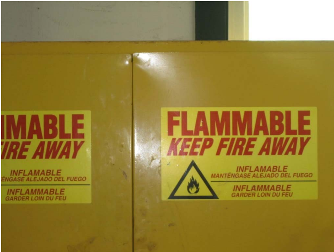
Photograph No. 6: Flammable cabinets, several throughout the shop.
