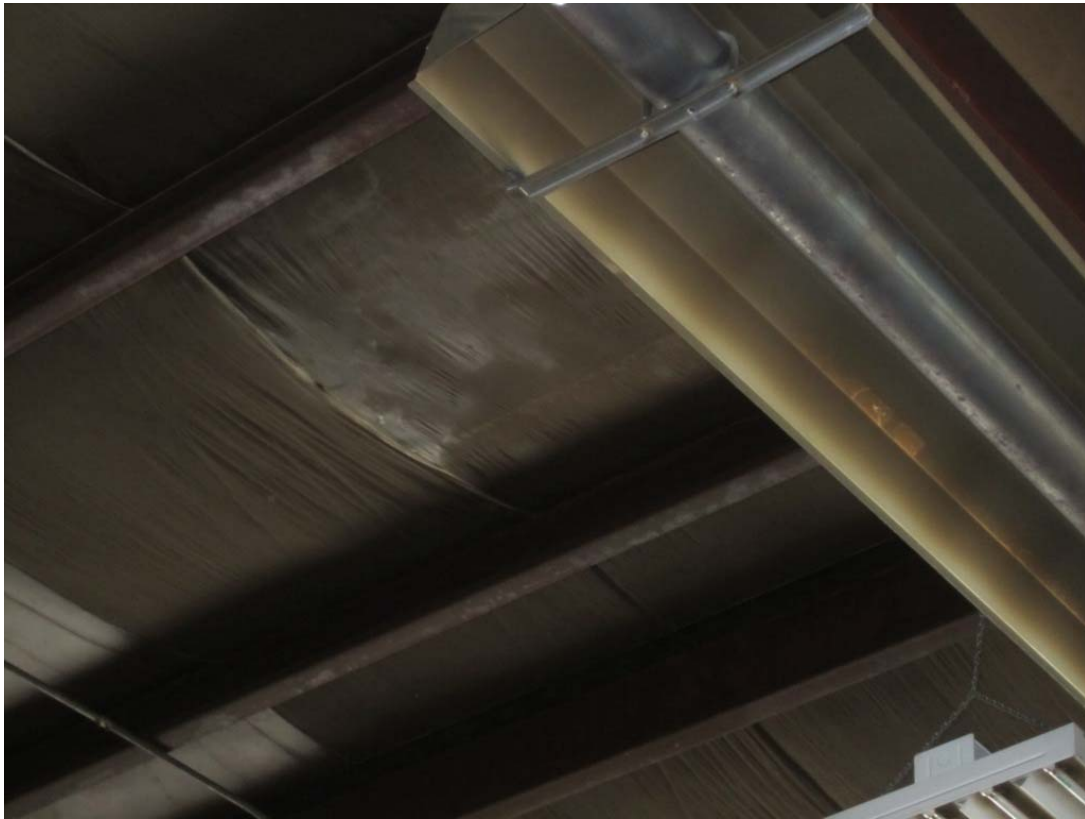
Photograph No. 11: Standard metal building insulation soaked by leaking roof.
