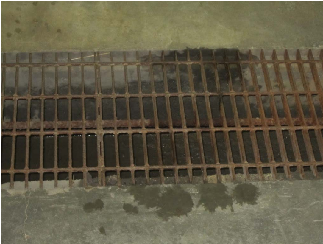
Photograph No. 20: Continuous floor drain grate to nowhere.
