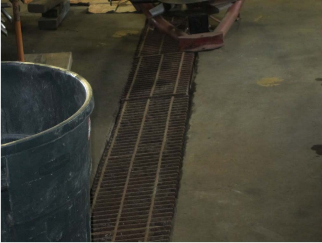
Photograph No. 7: Continuous floor grate for floor drain.
