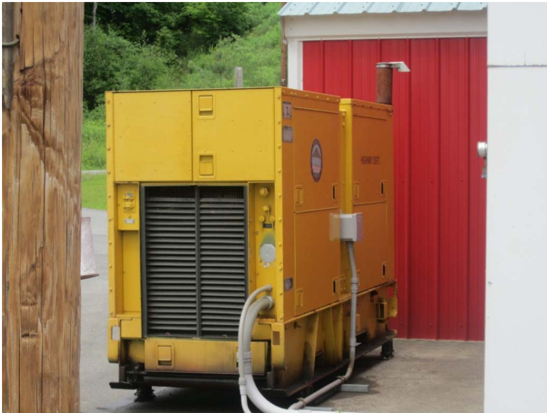
Photograph No. 12: Generator
