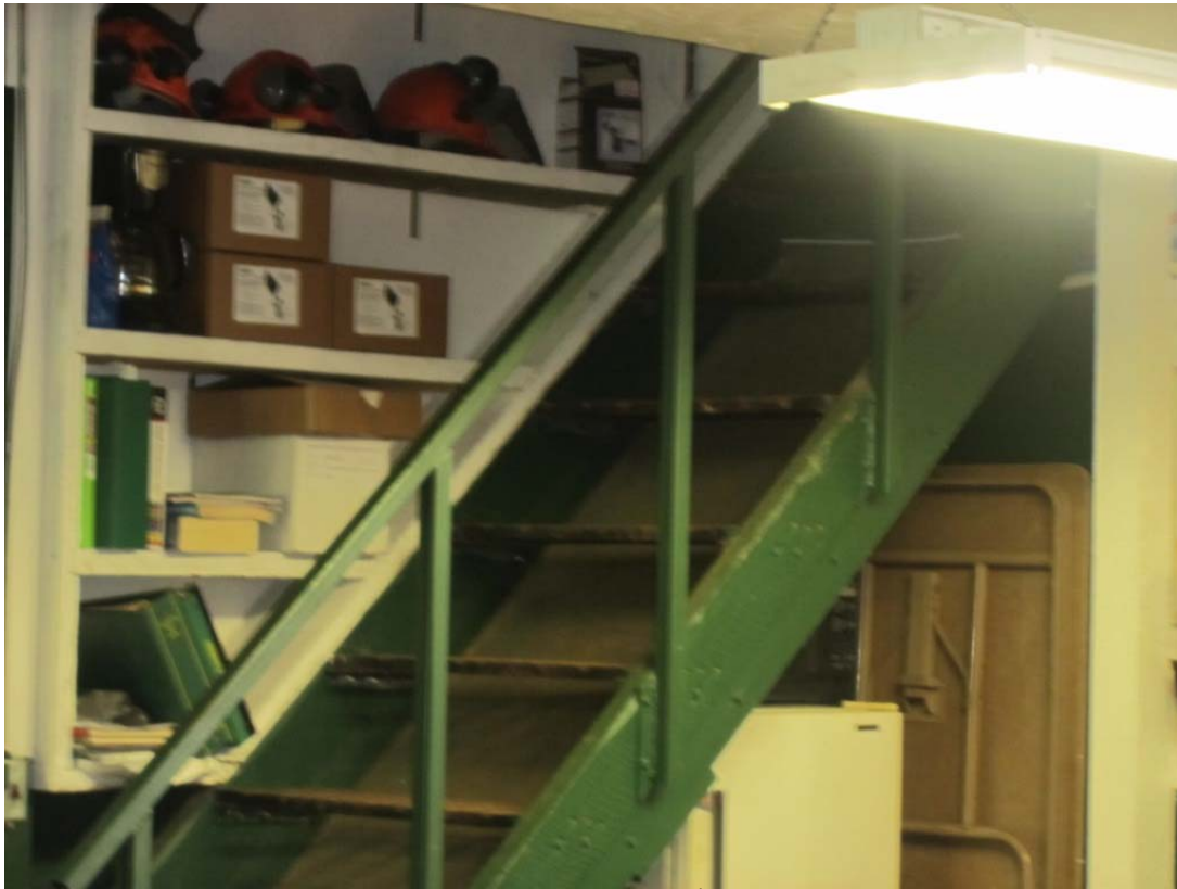
Photograph No. 5: More of the stairway to the 2 nd level that needs mid-rail.
